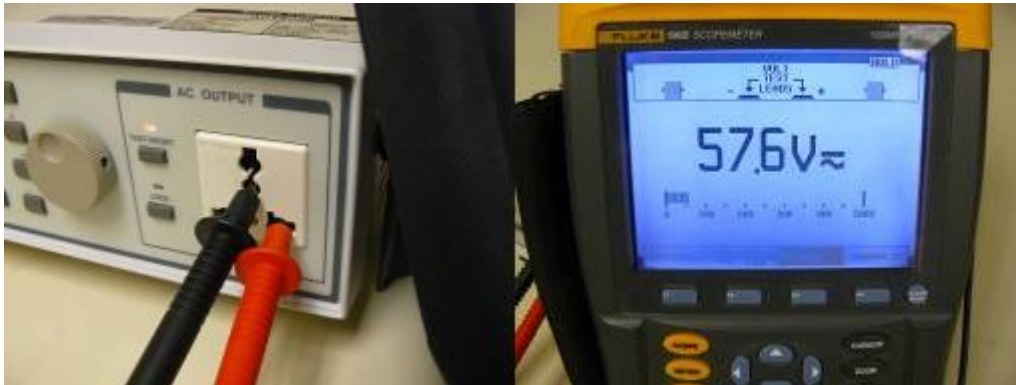
Figure 6c: Voltage measurement between neutral and ground
