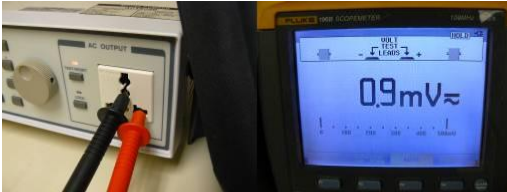
Figure 6c: Voltage measurement between neutral and ground with neutral tied to ground reference.
